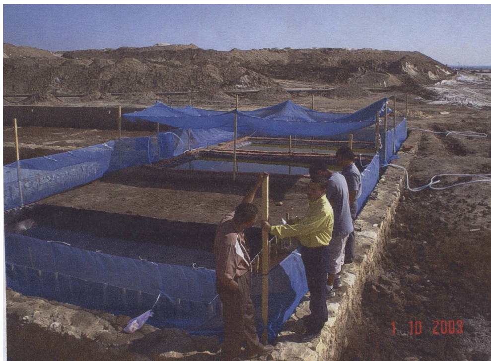
Plate (2): Ponds construction: under shade c-pond 2, beside shade c-pond1 and the other c-pond 3 [Emisal].
